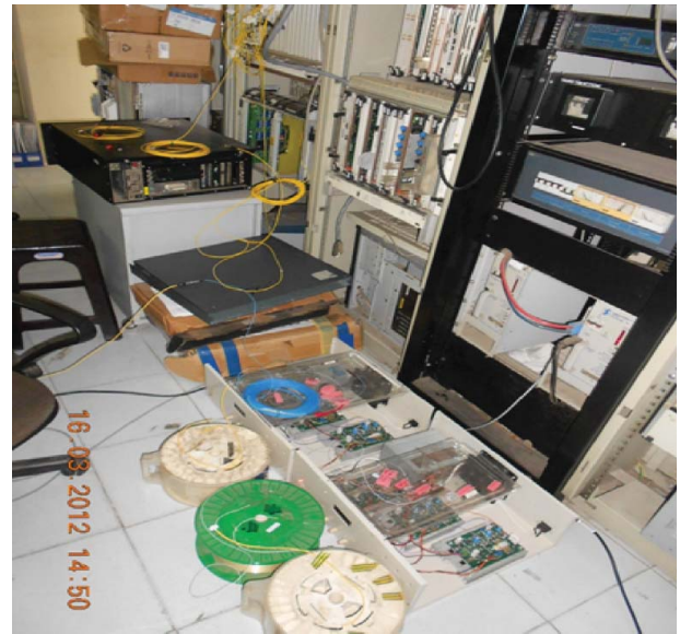
Figure 6: Raman amplifier on the DWDM system.
